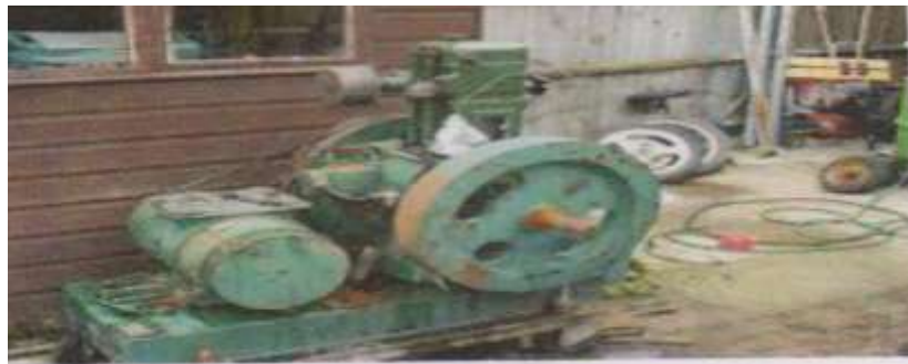
Fig. Dynamo connected with a diesel generator set.
