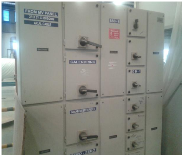
Switch ON the Main power
