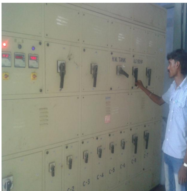
Switching on the main power panel
