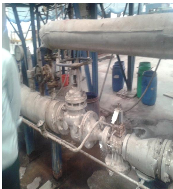
Opening Steam, water and air valve
