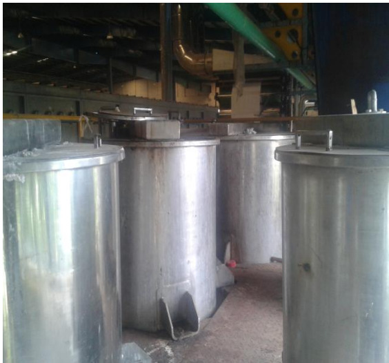
Caustic soda tank
