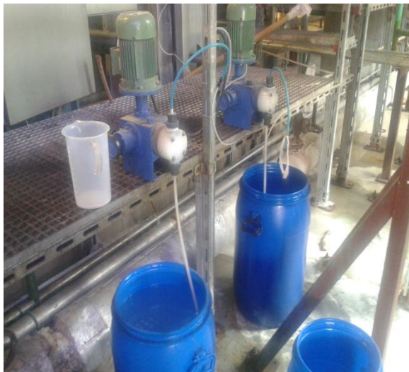
Acid dosing system
